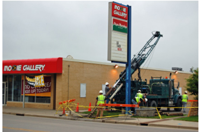
Seven remediation wells were drilled in August 2009 beneath Main Street between First and Second Avenue NW. The wells extend at a slant from south of Main to the center of the street, an area not previously reached for clean-up.
