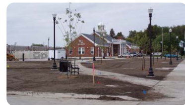
Reconstruction of a three-block area on the south side of Main Street includes a public square for expanded downtown activities, landscaped parking areas and space reserved for future commercial development.
