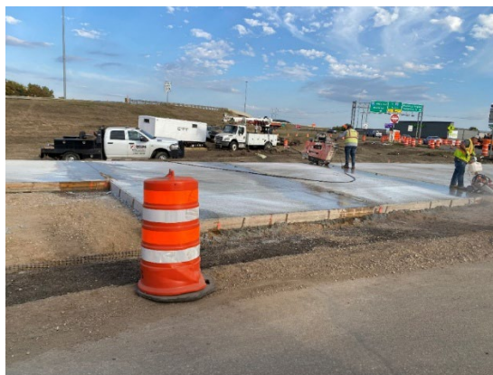
Photo showing concrete paving at 46th Avenue and Memorial Highway intersection, taken on September 11, 2025.
